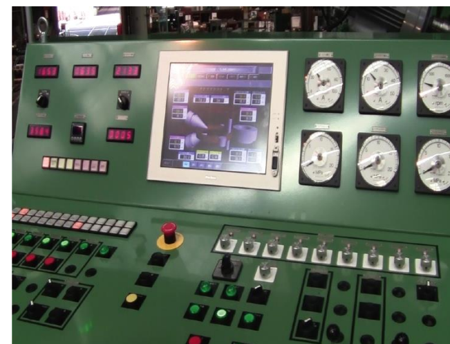
操作盤 Control Board
